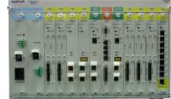
SDH transmission multiplexer
